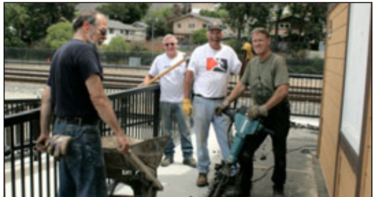
Glen Matteson, Tom Cooper, Tom Mitchell, and Brad LaRose breakup and remove old asphalt deck on the platform.
