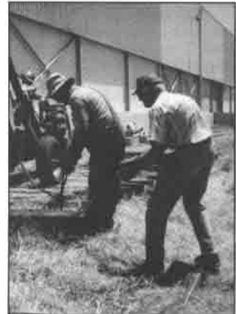
Andy McMeans and Arnold Jonas wrestle ties out of roadbed while Brad LaRose maneuvers tractor.
