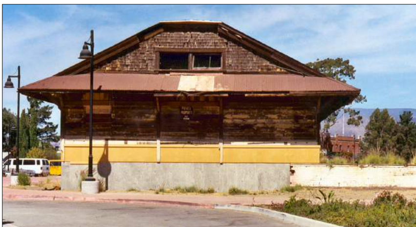
The Freighthouse when it was being restored. We've come a long way, but maintenance needs continue. Photo from SLORRM collection.
