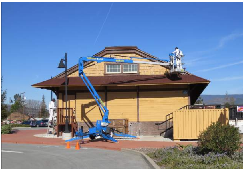
Browder Painting's crew works on the south end of the Freighthouse under City of San Luis Obispo contract. Photo by Glen Matteson.
