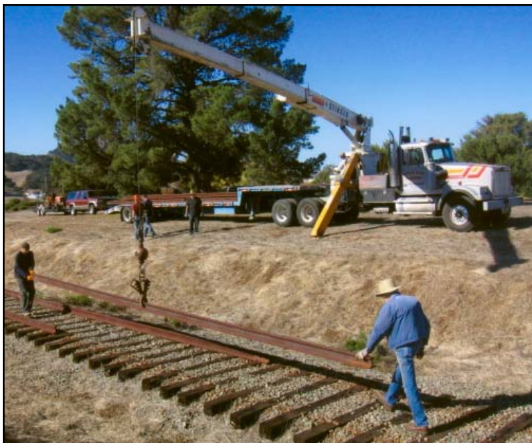
Arnold Jonas, in the foreground, guides a rail being lifted by Superior Crane to the truck in the background for transport to the Museum site.
