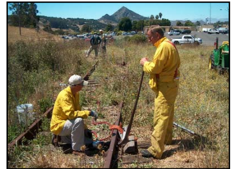
Howard Amborn, kneeling with impact wrench, and Ted VanKlaveren, with a spike puller, remove a stubborn nut from a rail-jointer plate.
