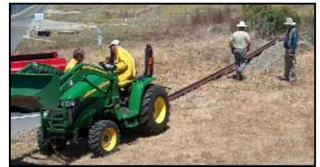
Howard Amborn uses his helpful tractor to pull a length of rail from the old right-of-way to a spot next to the parking lot for loading and moving to the Emily Street Yard.
